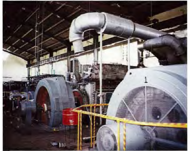
Vista interior de la Central Térmica de Taparachi. Internal view at the Taparachi Thermal Power Station.
