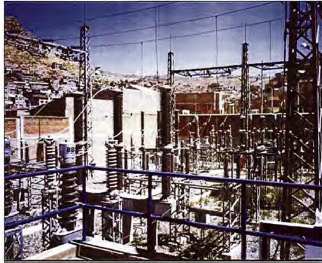
Patio de llaves C.T. Bellavista. Switchyard at the Bellavista Thermal Power Station
