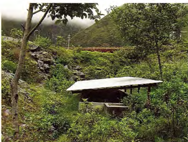
Pozo séptico Villa de Residentes. Earth filling at the Resident Village's installations.
