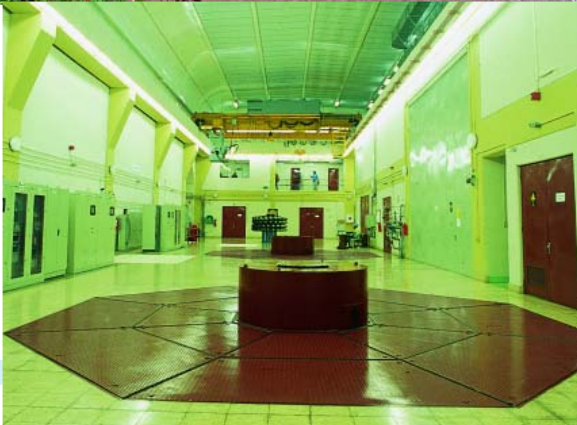
Casa de Máquinas CHSGBII Nivel Principal. Generadores 1 y 2 Power House San Gabán II Hydroelectric Power Plant. Main Level and Generators 1 and 2.
