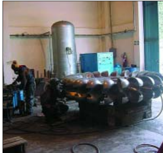
Esmerilado y Pulido de las cucharas del Rodete Pelton Sanding and finishing of the Pelton Runner buckets
