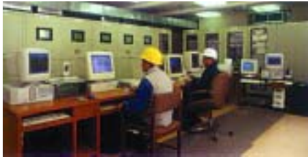
Centro de Control SE. SGBII Control Center Sub-Station SGBII
