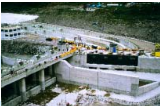
Lote 1: Obras Concluidas de Cabecera de la C.H. San Gabán II Lot 1 - Concluded Head Works of the San Gabán II Hydroelectric Power Plant
