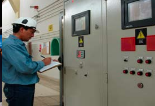
Operador C.H. san Gabán II Technical Operator at San Gabán II Hydroelectric Power Plant
