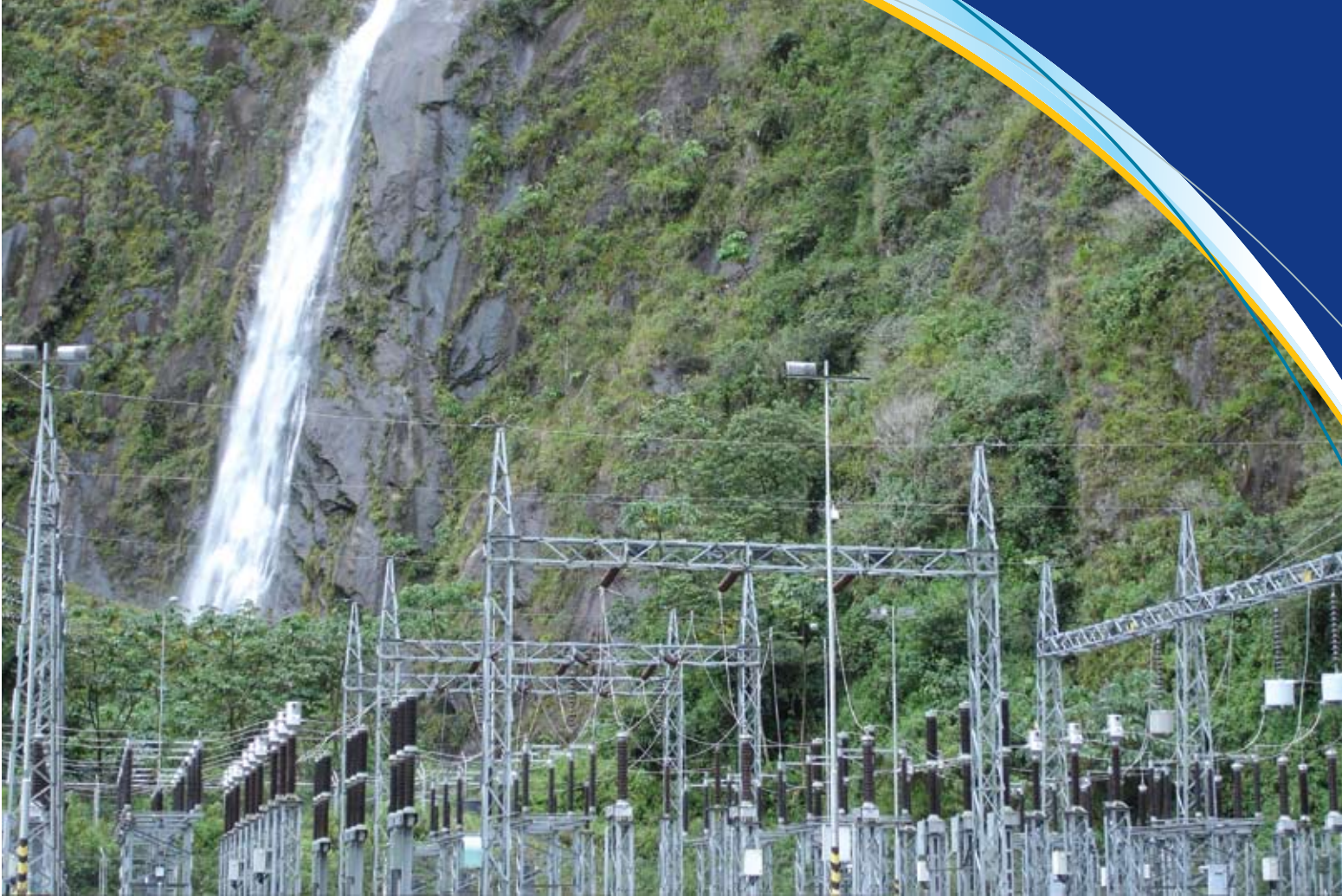
Patio de llaves S.E. San Gabán II Switchboard yard Sub Station, San Gabán II
