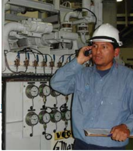
Operación C.H. San Gabán II Operation activities in San Gabán II Hydroelectric Power Plant
