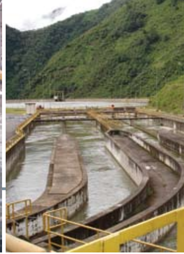
Naves desarenadoras C.H. San Gabán II Water settlement ponds, San Gabán Hydroelectric Power Plant
