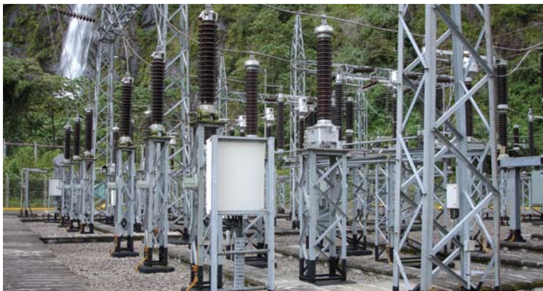
Patio de llaves S.E. San Gabán II / Switch board yard at San Gabán II Hydroelectric Power Plant
