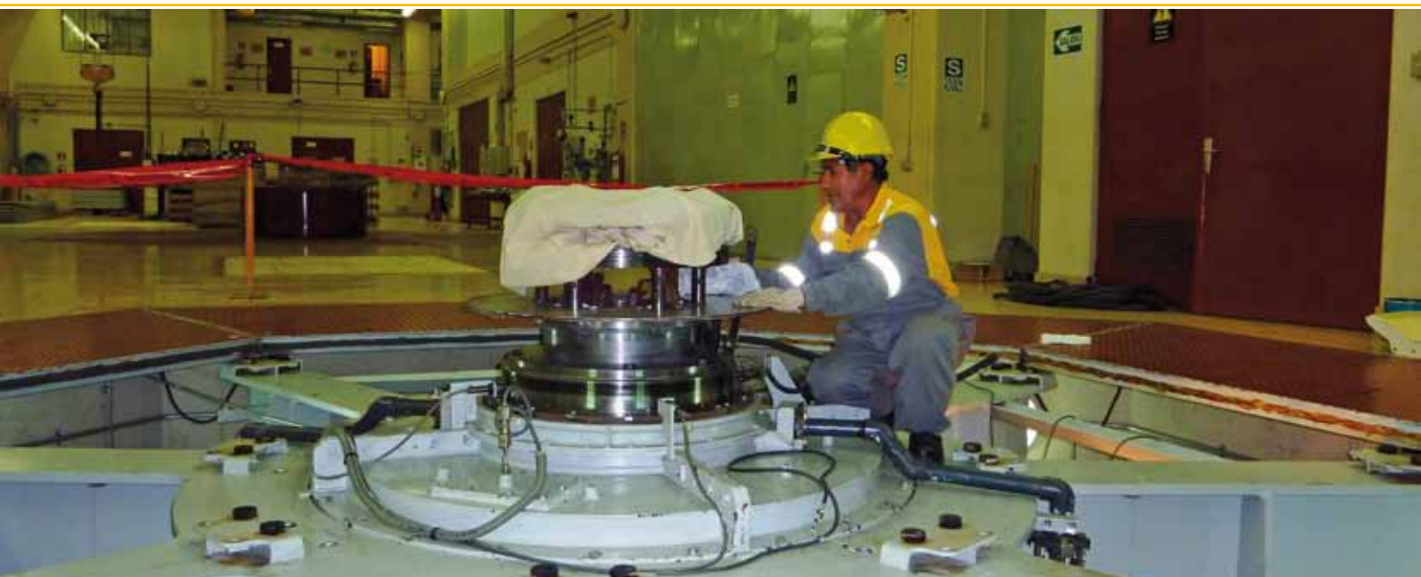
Mantenimiento de alternador C.H. San Gabán II / Alternator maintenance at San Gabán II Hydroelectric Power Plant
