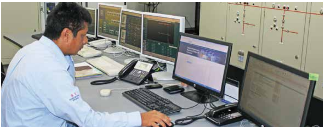
Centro de Control C.H. San Gabán II / San Gaban II Hydroelectric Station Center of Control
