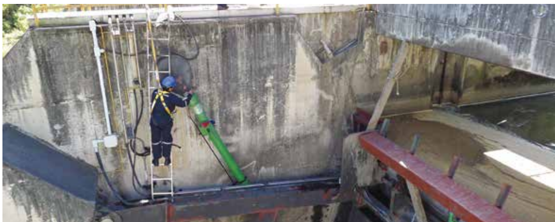
Mantenimiento de Compuertas C.H. San Gabán II / San Gabán II Hydroelectric Station gates maintenance
