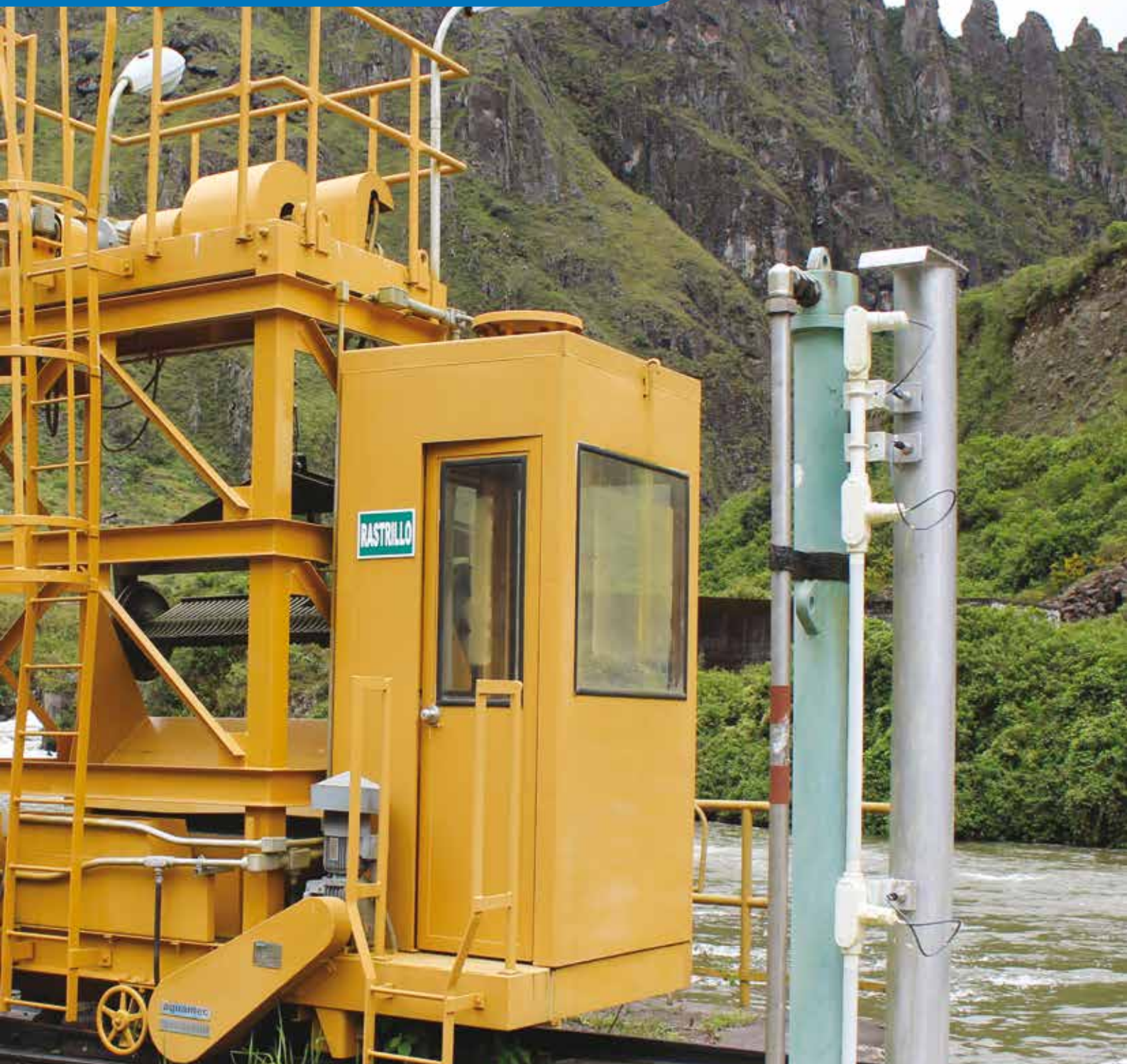
Rastrillo de limpieza Bocatoma C.H. San Gabán II / San Gaban II Hydroelectric Station intake rake
